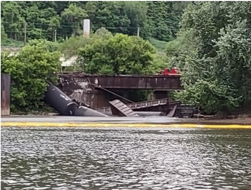
Photo of Train Derailment in Harmar, PA from May 2022 (Credit: Three Rivers Waterkeeper)
